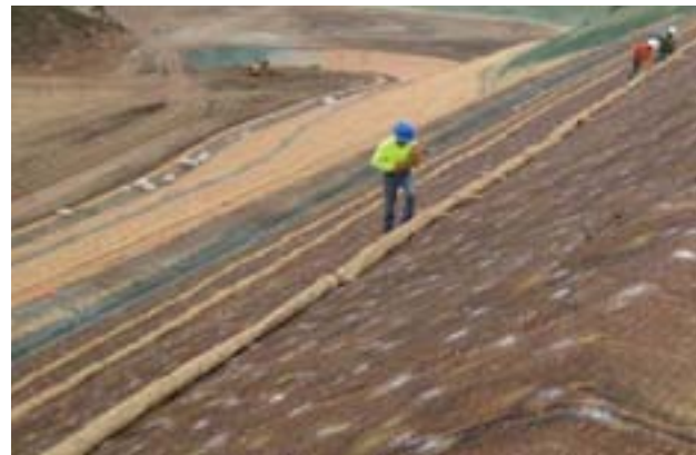
The RollMax TRMs are installed in a one-step operation directly over the prepared seedbed saving time and money and ensuring the highest level of erosion control and vegetation reinforcement.
